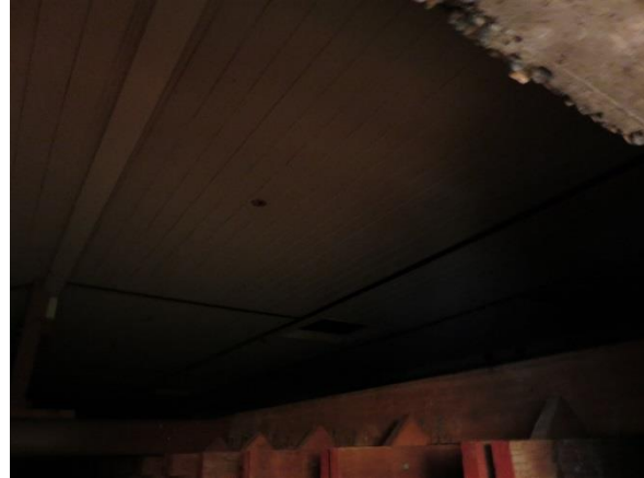
Figure 3.46 The original boarded ceiling remains above the newer cedar ceiling in the chapel. The dark lines possibly indicate the former location of walls. (Source: GML 2017)
